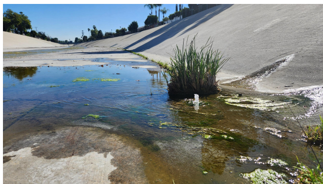
Fig. 4. Groundwater seepage through the concrete lining in the Upper Los Angeles River.
