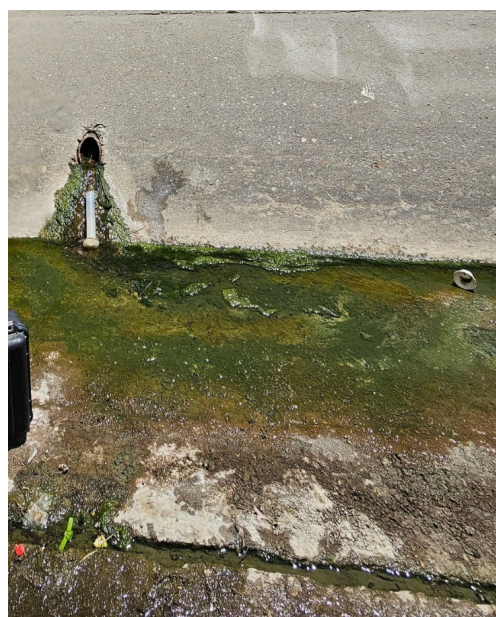
Fig. 8. Weephole (S-Spring St.-WH4) at the southern end of the sampling area along the Lower Los Angeles River, illustrating groundwater seepage observed in this reach.
