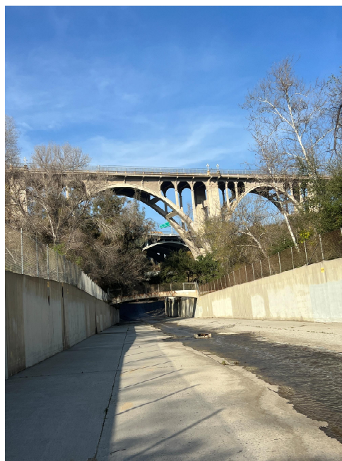
Fig. 6. Lower Arroyo Seco – Below the Colorado Bridge, the picture captures the drop-off marking the start of the channelized reach where groundwater seeps in through weepholes, French drains, and cracks in the concrete.
