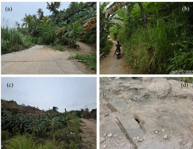
Fig. 7. Post-failure access and surface deformation (a) narrow improvised bypass at the failed section; (b) motorcycle crosses toward Barangay Fatima; (c) unpaved track with banana regrowth on the slide mass; (d) developing tensile crack along the path.
