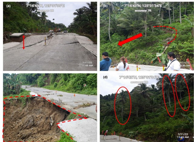
Fig. 4. Indicators of slope instability (a) roadway settlement & longitudinal cracks; (b) upslope tensile cracks; (c) downslope slip exposing cross-drain; (d) leaning trees (creep).
