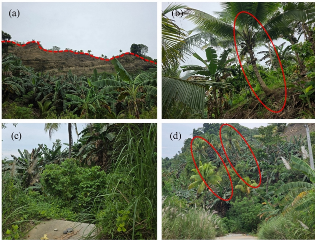
Fig. 6. Ongoing slope movement indicators (a) main scarp with banana regrowth, (b) leaning coconut with exposed roots, (c) displaced pavement at one end of the collapsed road, and (d) bent trees downslope.
